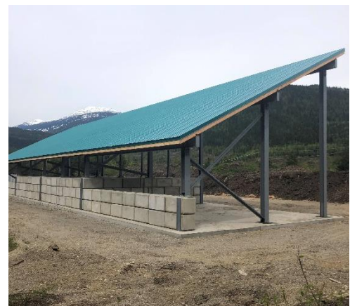
Figure 17 Compost bunkers for receiving and mixing at the Revelstoke composting facility
