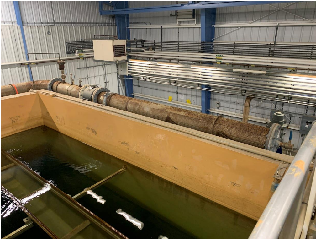
Figure 6: Corrosion of Existing Stainless Steel Piping
