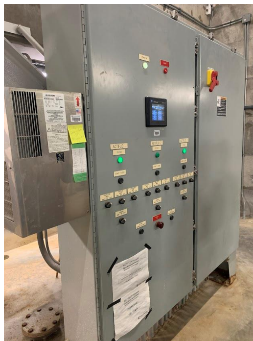
Figure 4: Existing Actiflo® Control Panel
