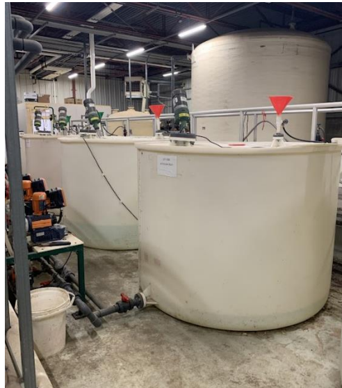
Figure 3: Existing Deep River WTP Actiflo® Polymer Manual Mixing Equipment
