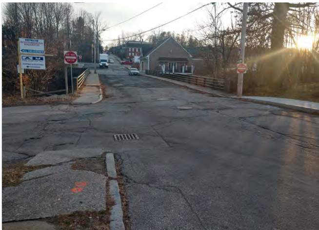
The River Street Bridge provides a convenient way to cross the Quinebaug River.
