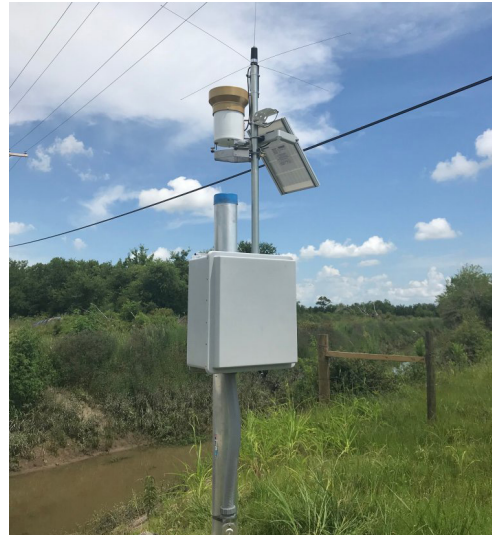
Image: Calcasieu Parish Gauge in Kayouche Coulee Watershed
