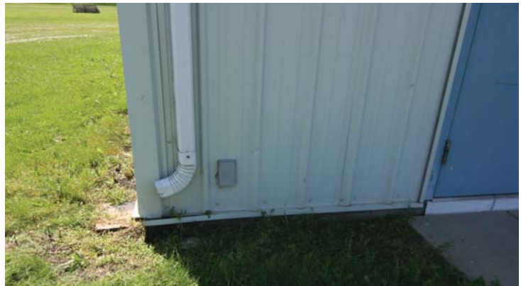
Currently there is not positive drainage away from the building.
