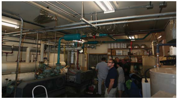
Service Room and Ice Plant
