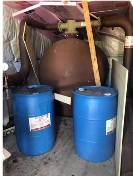
600-gallon foam concentrate tank and drums of AFFF
