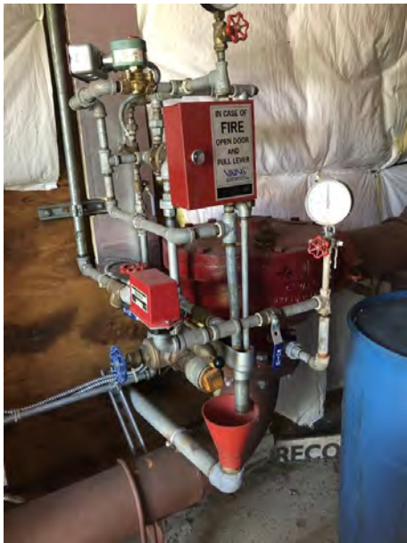
Foam system emergency activation pull station
