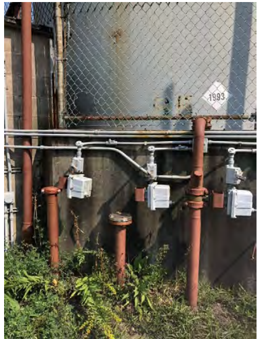
Fire suppression system piping
