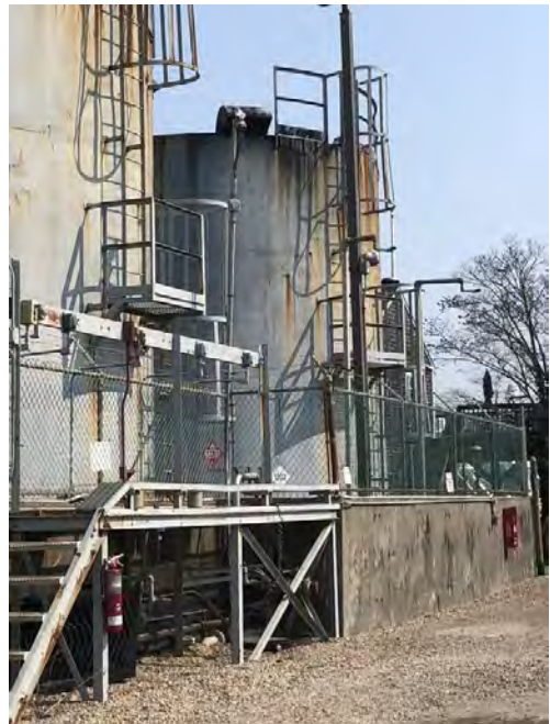
Fuel loading rack
