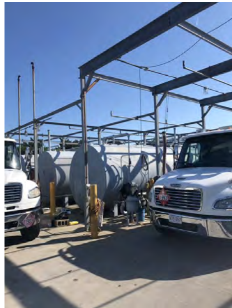
Fuel storage tanks and fire suppression system
