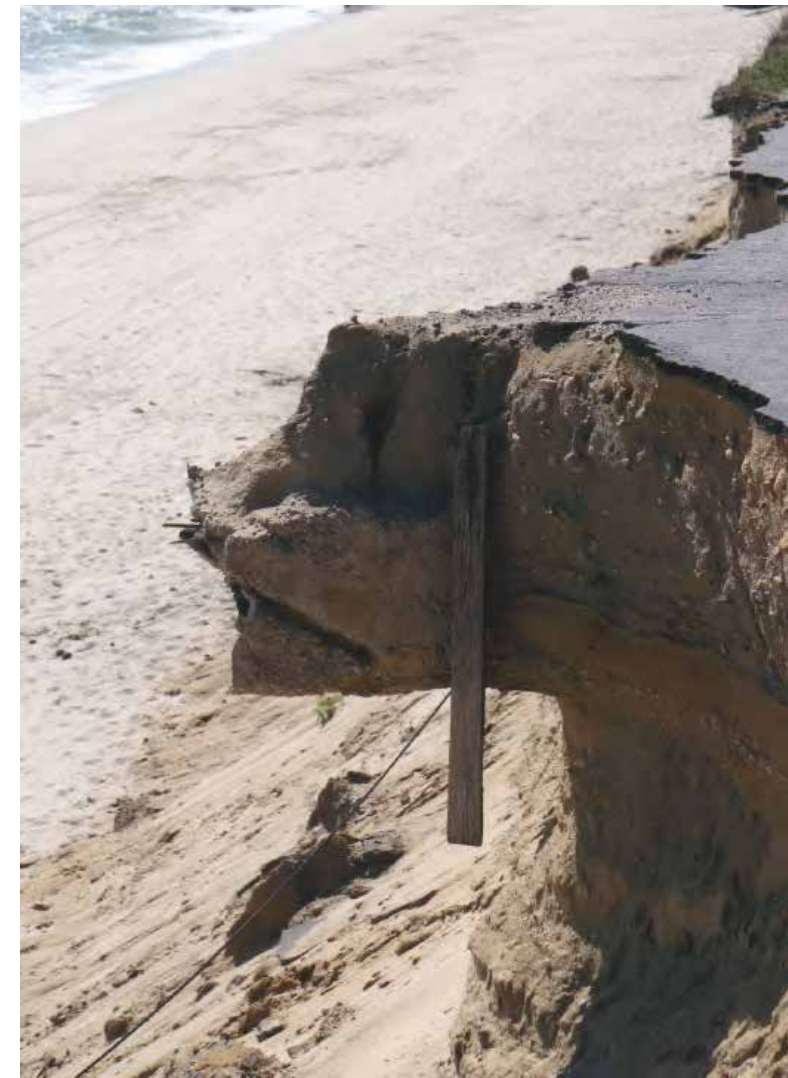
Erosion at Tom Nevers | September 2024
