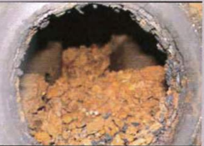
"In-tank" flue tubes and heat exchangers suffer from lime scale buildup beginning from the first hours of operation.
