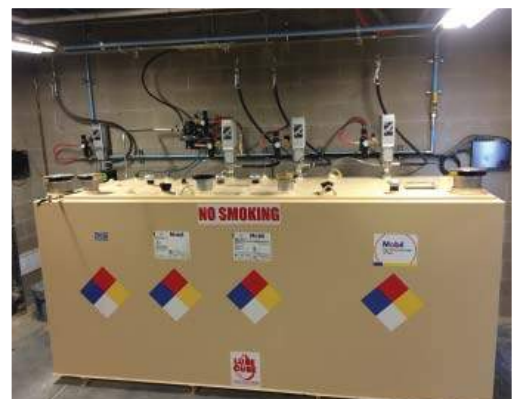
1,250 gallon, 4 compartment tank.
