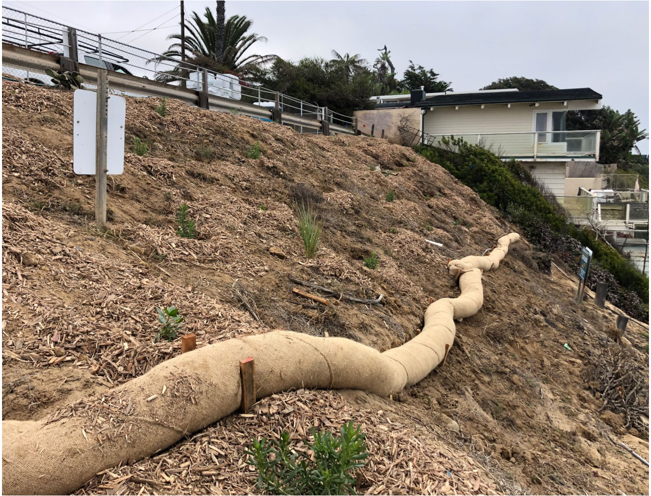
Rewilding at Beacons Bluff, showing erosion control and native plants being reinstalled to help reduce surface erosion.
