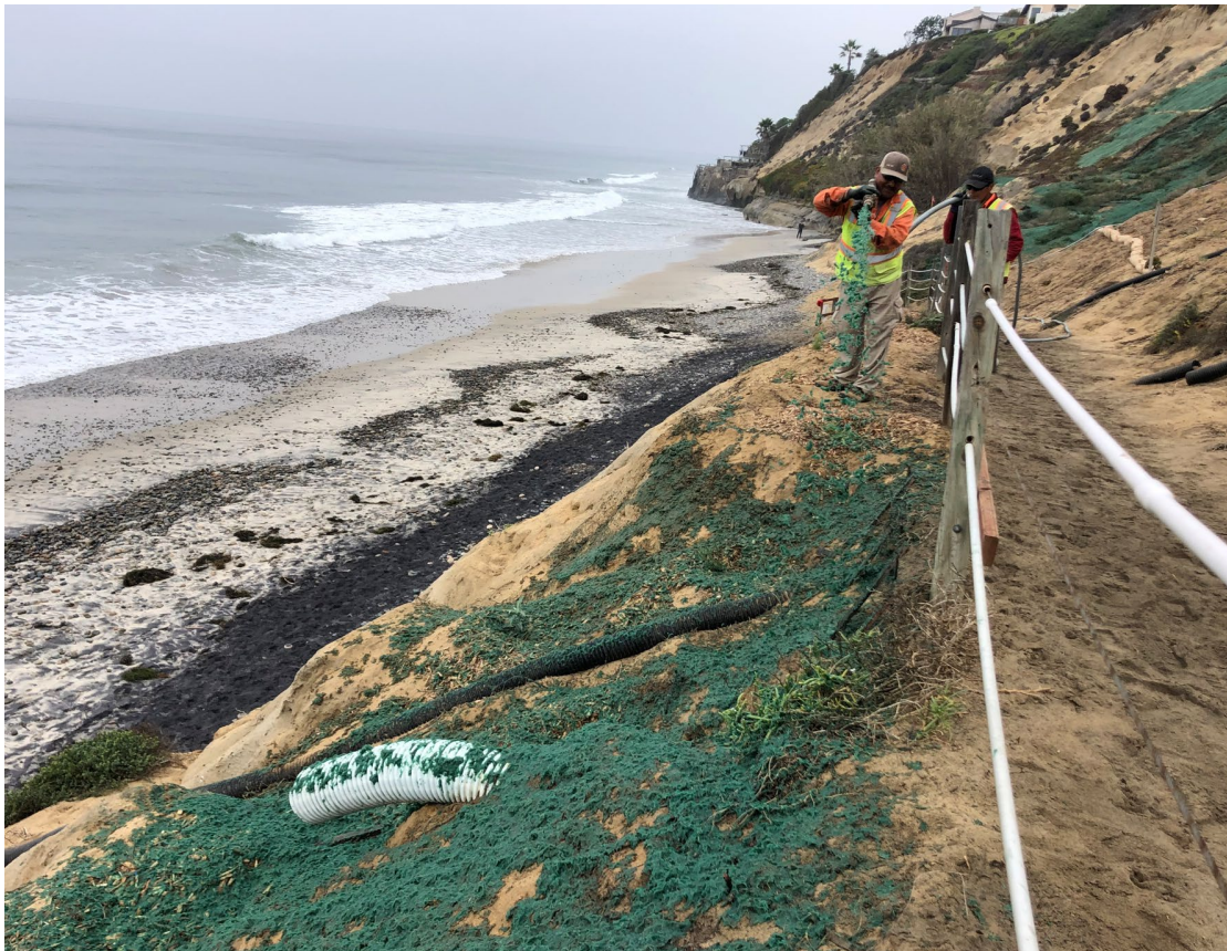
This photo shows an example of rewilding in Encinitas, using a native hydroseed bluff mixture to reduce surface erosion along Torrey Sandstone bluffs to help stabilize the bluff at as part of the Beacons Beach Landscape Restoration Plan.
