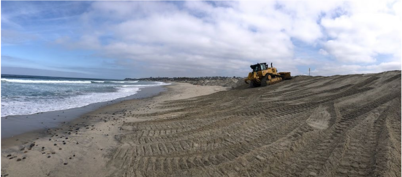
Maintaining the Cardiff State Beach Living Shoreline after the 2024 El Nino storms.
