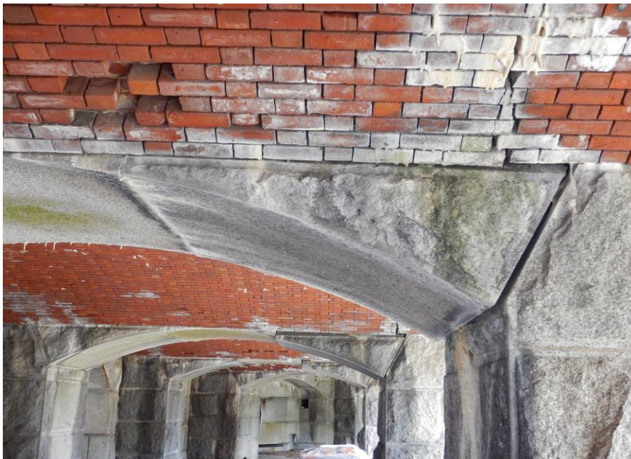
Top photo: First Tier circumferential crack; bottom photo: Second Tier circumferential crack.
