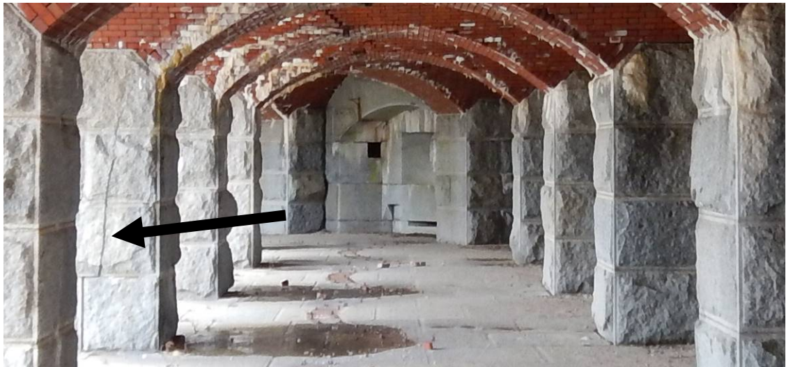
Crack in First Floor Casemate Pier on Parade Ground Wall
