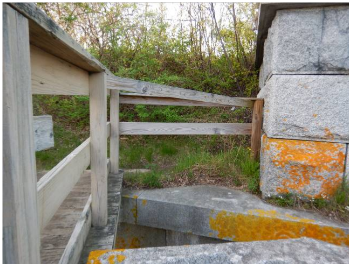
Photo 4.8 Unsafe Railing System at Barbette Tier Bridge and Path
