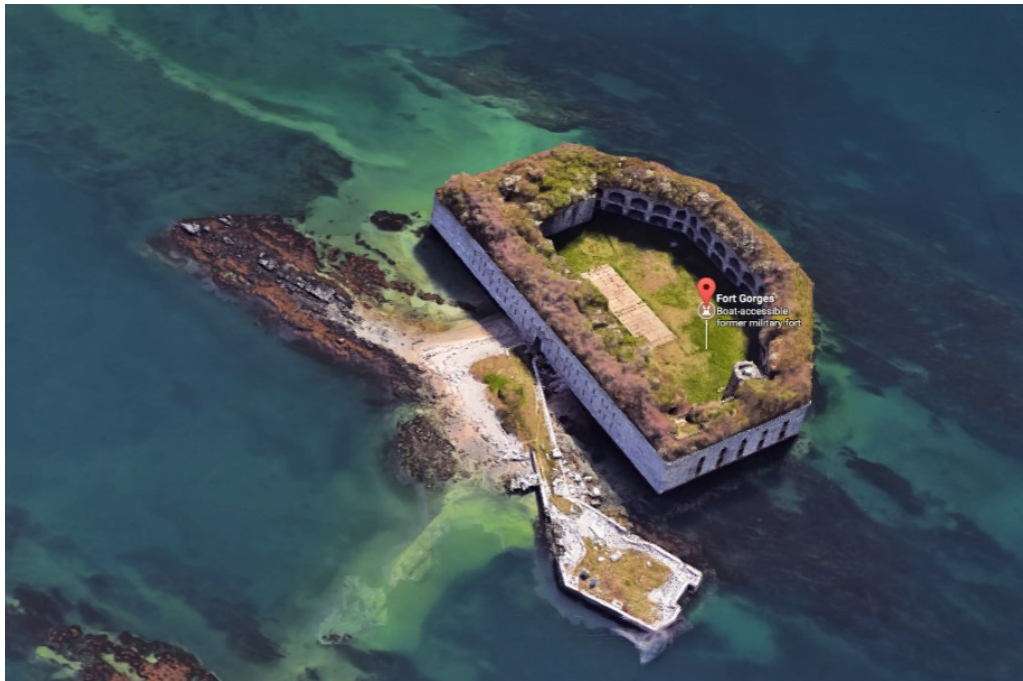
Wharf Structure, ravaged by tides: Top Photo HABS No. ME-134-23; Bottom Photo, Google Earth
