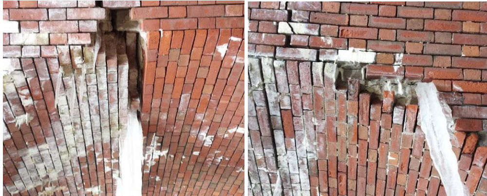
Typical First-Tier Casemate Damage along circumferential cracks and arch intersections.
