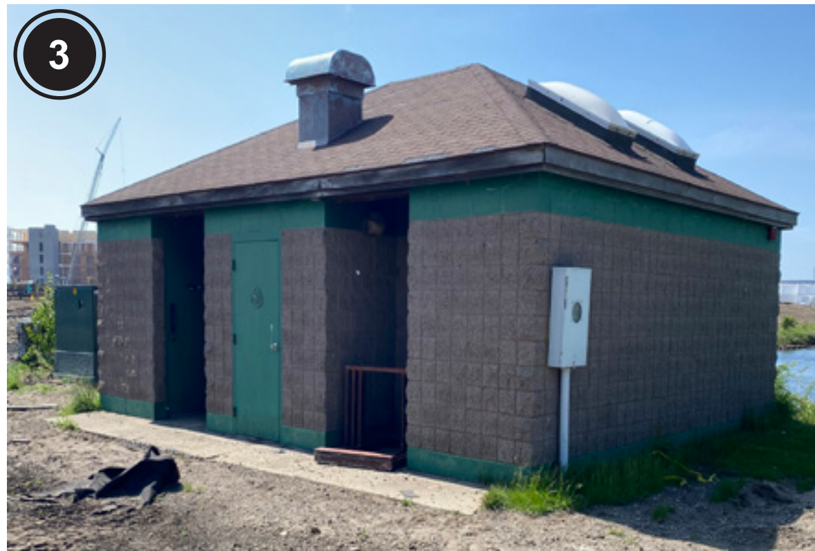
3 EXISTING RESTROOM BUILDING REQUIRES REPAIRS OR REPLACEMENT
