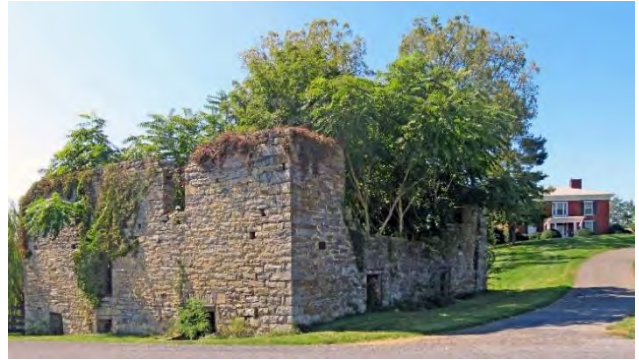
Bare House (background) and Mill ruins (foreground), Virginia Department of Historic Resources
