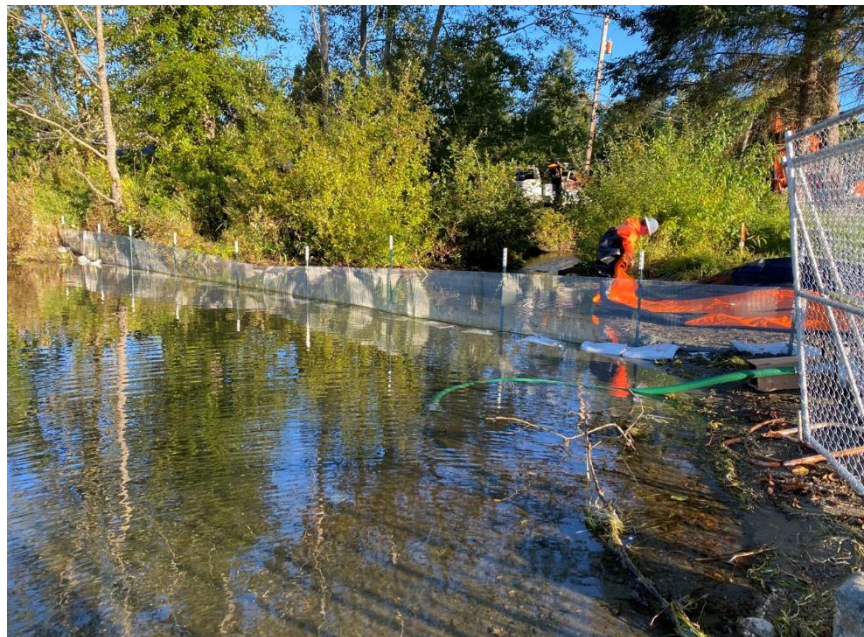
Figure 9 photograph at the mouth of the Lake Outlet (looking downstream) prior to dredging as cofferdam and bypass pumps are installed.
