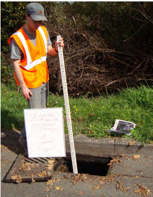
Photo 4. Catch Basin on NE 125th Street on East Side of Street nearest intersection with 18th Avenue NE on September 25, 2019.
