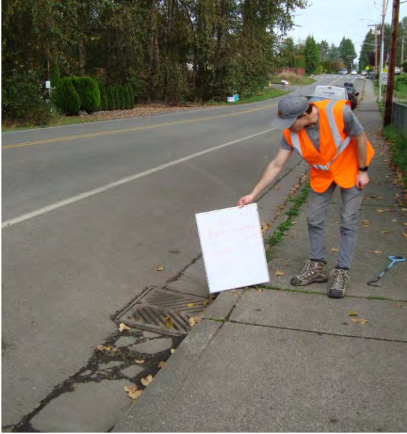
Photo 8. Catch Basin at low point on 20th Avenue NE near culvert crossing.
