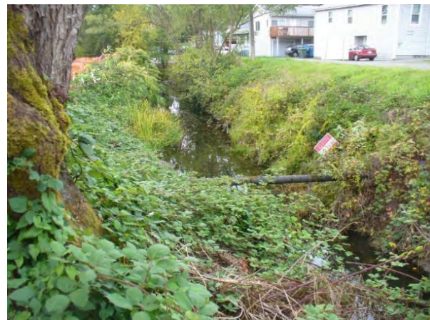
Photo 18. Facing upstream, channel section along N. Lakeshore Dr. Note elevated sanitary sewer crossing and invasive vegetation. Extensive bank armoring is obscured by shrubby vegetation. 10/3/19
