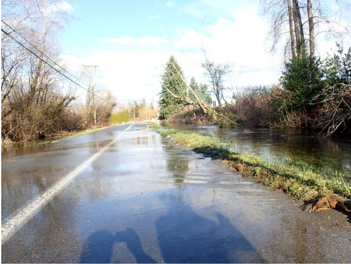
Photo 14. Hartford Drive in the vicinity of historic outlet channel on February 11, 2020. Hartford Drive was closed due to water over the roadway (approximately 1.5 inches deep on 2/11/2020).
