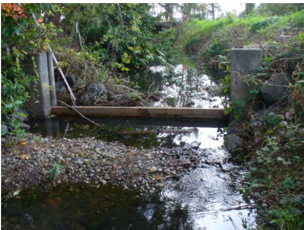
Photo 17. Existing lake outlet control weir is manually-operated. It does not regulate low flows well due to leakage and may be an upstream fish passage barrier during low flow periods as well. 10/3/19
