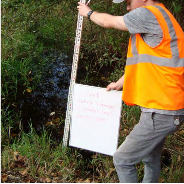
Photo 12. Conveyance ditch downstream of culvert crossing on north side of 20th Avenue NE.
